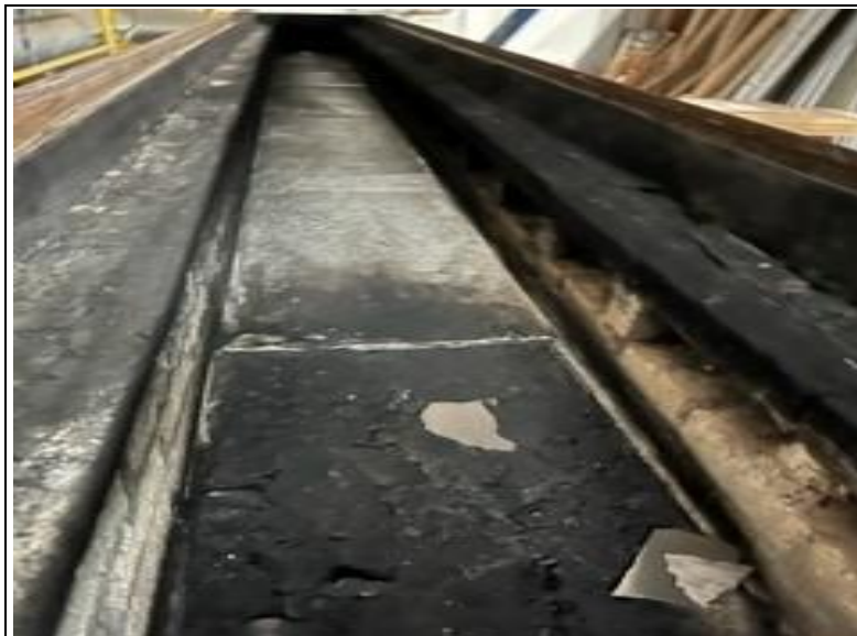
Photo No. 2 Post Test
